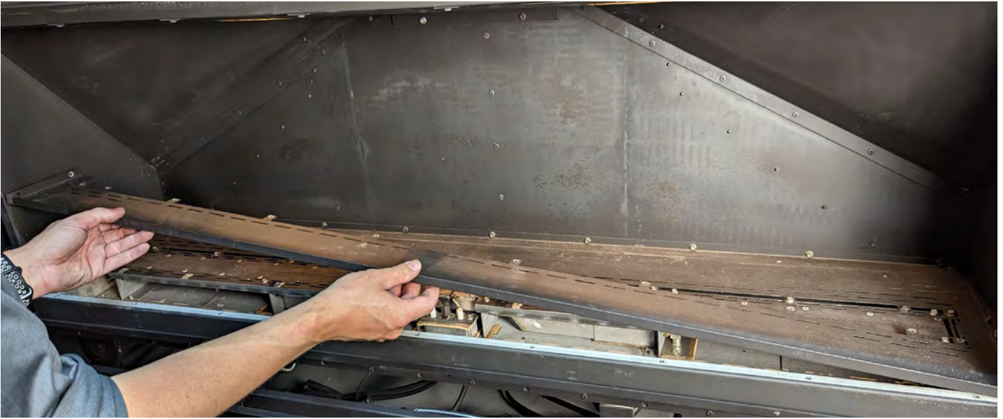
Figure 18.13.03: Front of burner surround
