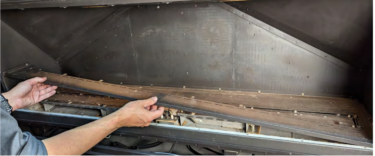
Figure 18.13.03: Front of burner surround
