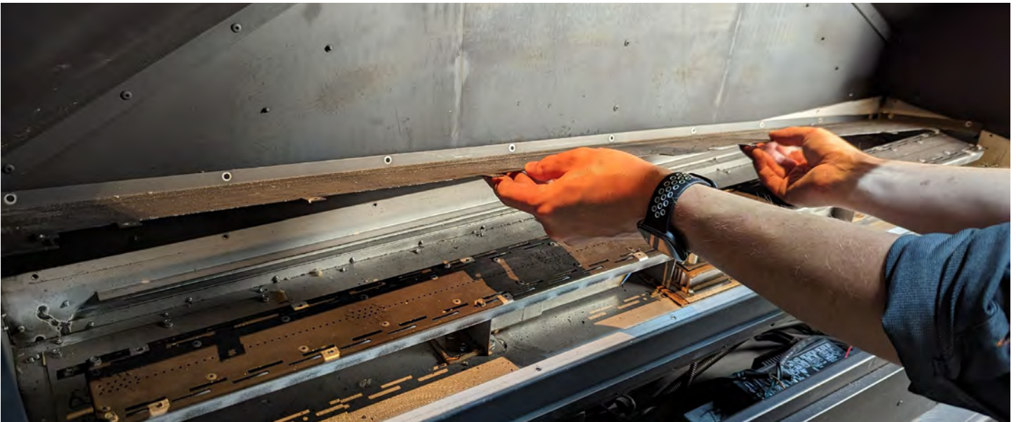
Figure 18.13.04: Back of burner surround
